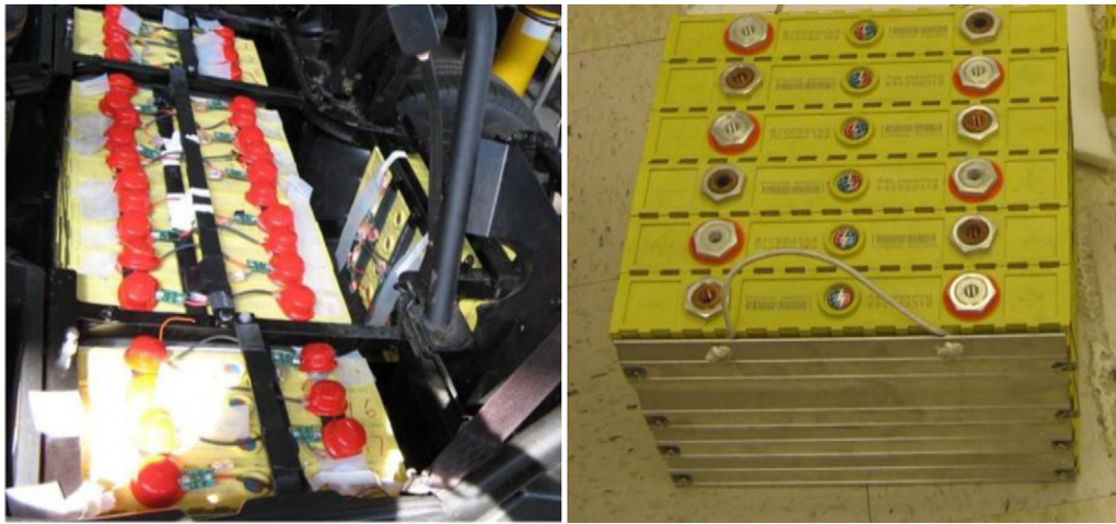
Fig. 2. Li-ion batteries installed on the FIAIWM EGV.
